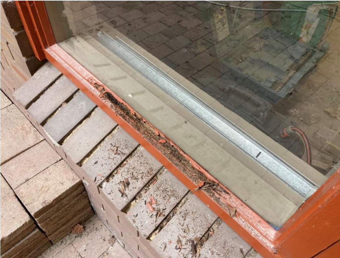
Window Framing Weather Damage and Rot
