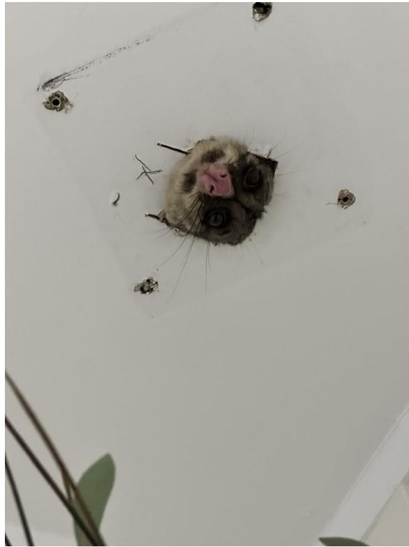
Holes in the ceiling
