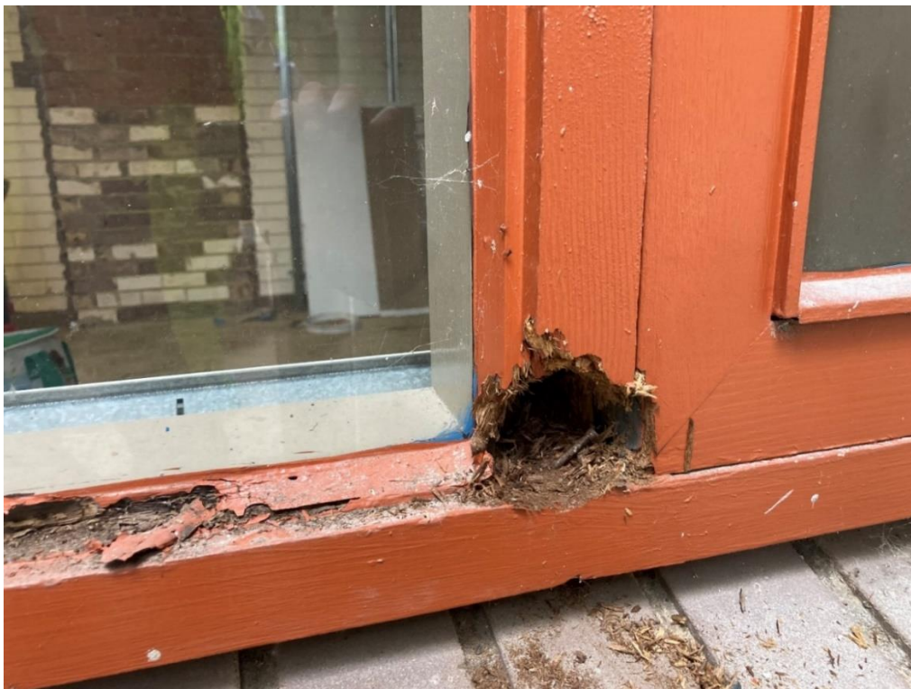
Window Framing Timber Rot and Weather Damage
