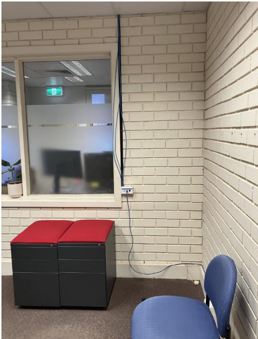
Poor Cable Management – Hook or Trip Hazard
