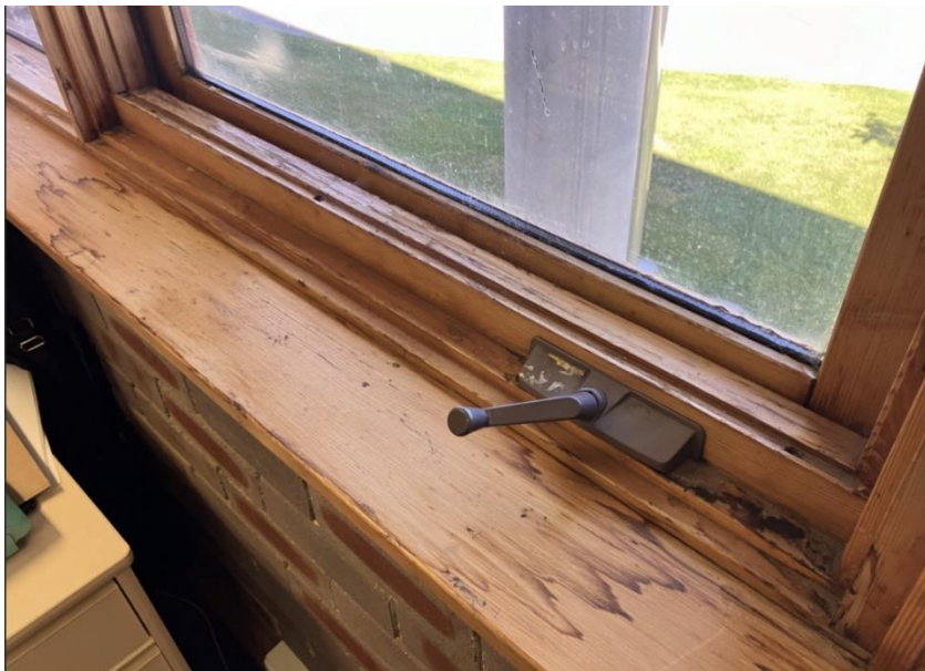
Water Damage internally suggesting water ingress through window framing
