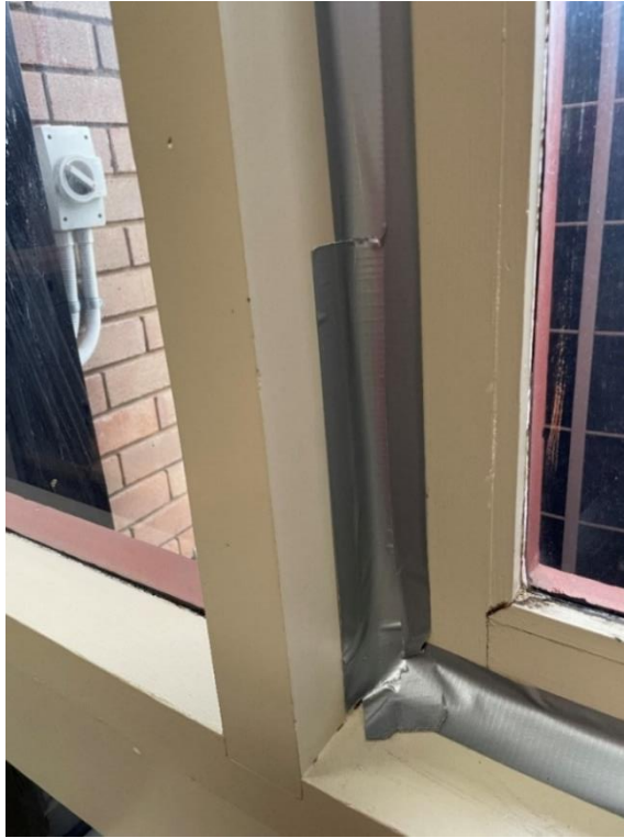
Windows sealed with tape to try and prevent draft and the cold coming in.
