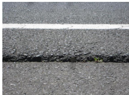
Figure 2.7: Road shoulder pavement level difference - Illawarra Highway at Sheepwash Road, Avoca
