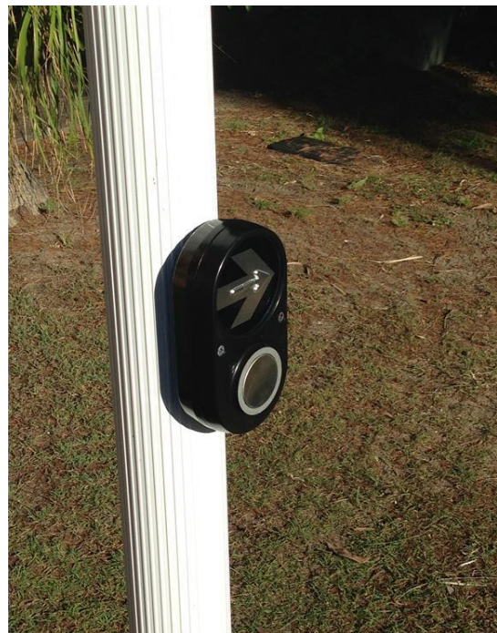
Figure 5.17: Bicycle activated warning sign push button – Noosa Parade, Noosa, Queensland
