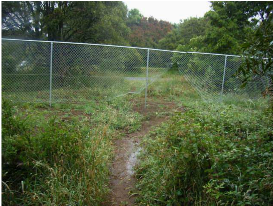
Figure 8: Hole in railway fence with clear "goat track"
