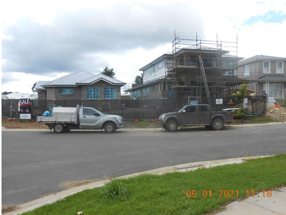
Photo 7: Shows elevation from Ginahgulla Drive of development under application 20/0720 for dual occupancy at 40 Sir James Fairfax Circuit Bowral
