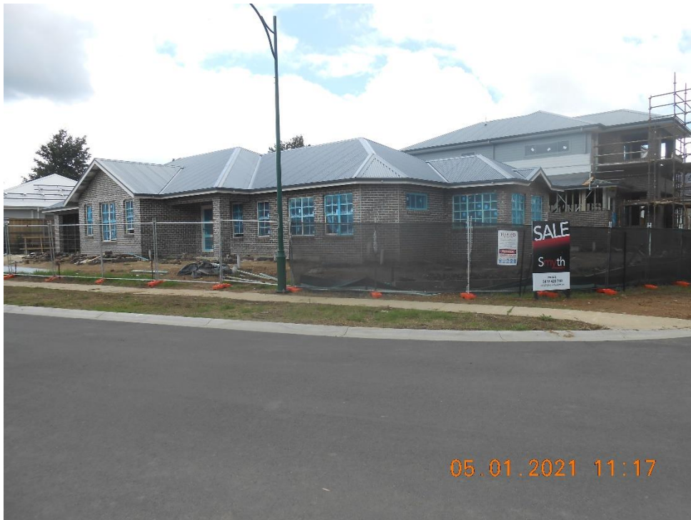
Photo 9: Shows elevation from Sir James Fairfax Circuit of development under application 20/0720 for dual occupancy at 40 Sir James Fairfax Circuit Bowral
