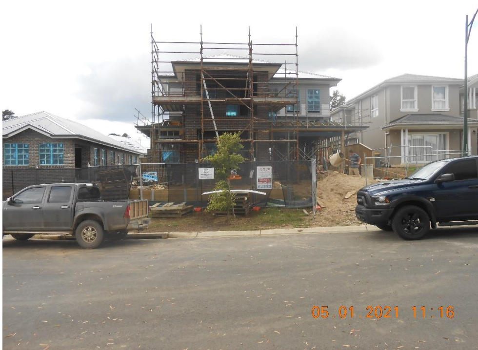
Photo 8: Shows elevation from Ginahgulla Drive of development under application 20/0720 for dual occupancy at 40 Sir James Fairfax Circuit Bowral
