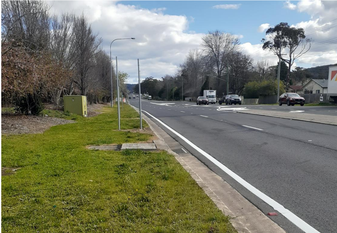
Image 2 – Recently completed road widening and traffic island facility opposite Rush Lane, Braemar
