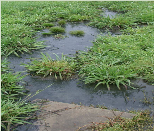
Example of a failing septic absorption trench
