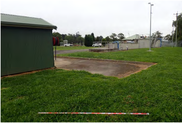
Plate 3: General location of where the revised pipeline will connect to subsurface, facing south.
