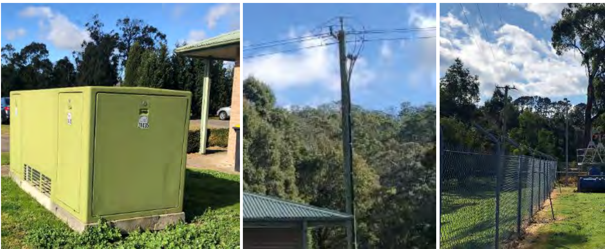
Figure 9-1 Existing Pad mount Substation, HV Connection & HV Powerline
