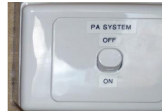
PA system switch
