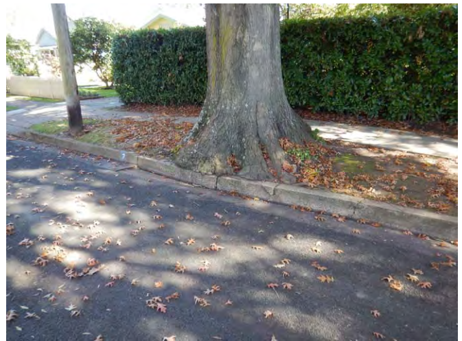
Figure 2.4 - A large tree in a narrow verge on Holly Street, Bowral increases the likelihood of damage to infrastructure and trip hazards in pavements. (Photo - Arterra)
